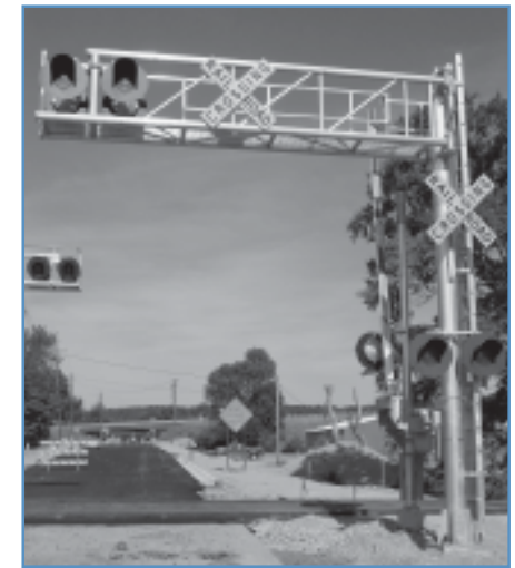
Resurfacing of the road and the new railroad crossing on Mt. Tabor Road.
